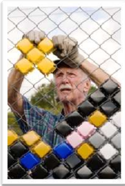
Bob Coffee and others helped to install the latest Art On the Way project
